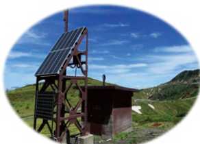
Borehole-type tiltmeter and seismometer station
