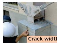
Damage reconnaissance of the 2016 Kumamoto EQ
